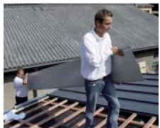
Transportation on the building site is no problem due to its light weight.
