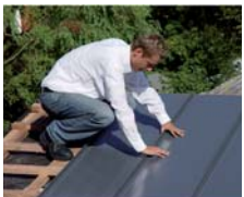
Place the next sheet on the prefabricated seam and clip it in.
